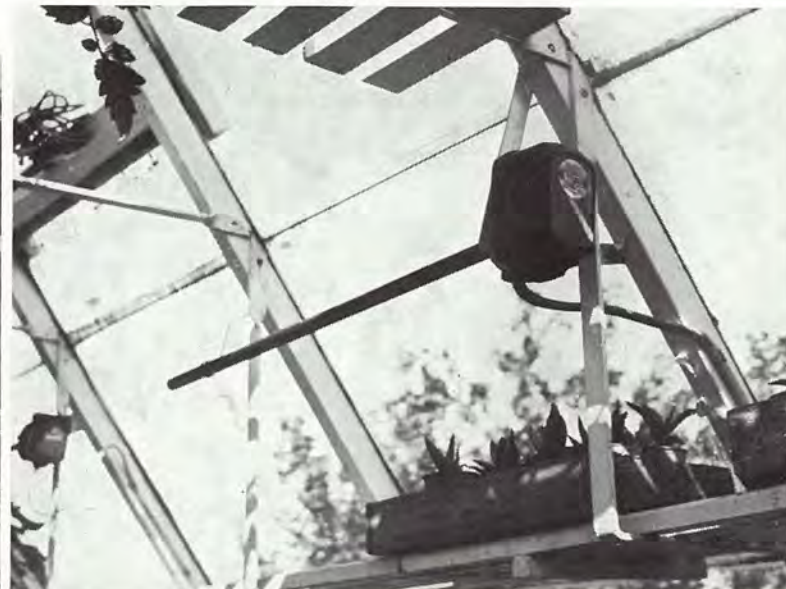
A 24-inch Proscen rod thermostat, correctly positioned.
