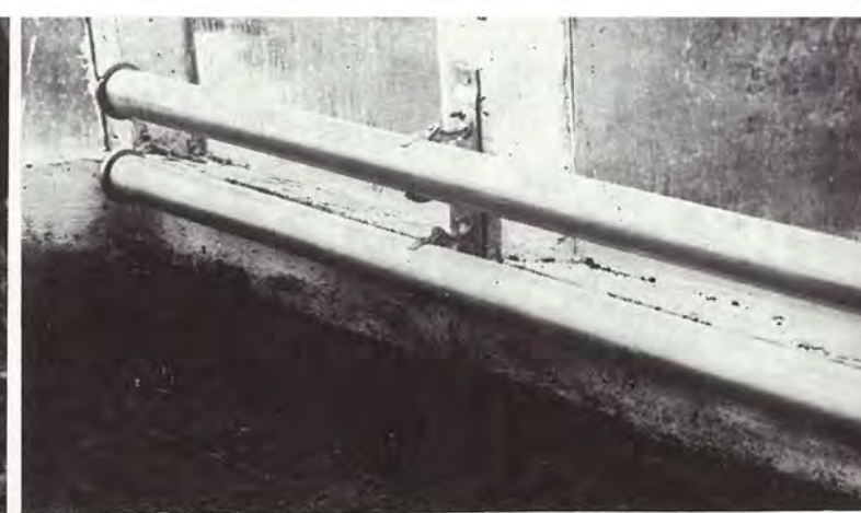
Tubular heating in a concrete greenhouse.
